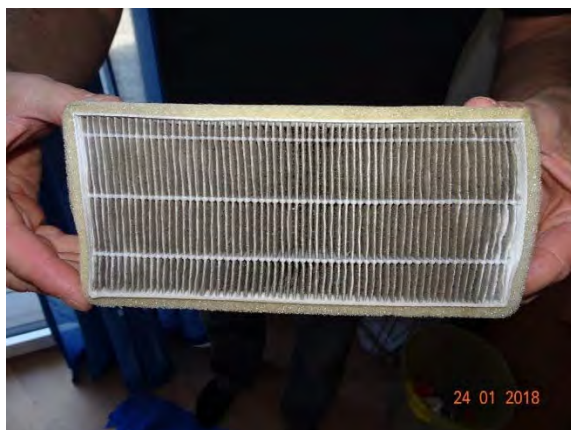
Abbildung 136: WNG ID 620: Zuluftfilter
