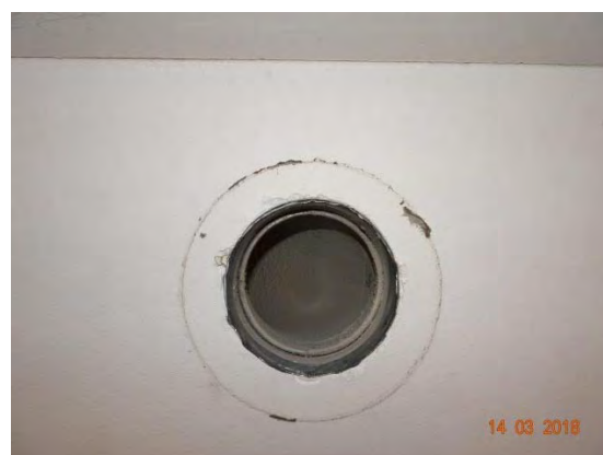
Abbildung 195: WNG ID 820: ABL-Rohr, Bad
