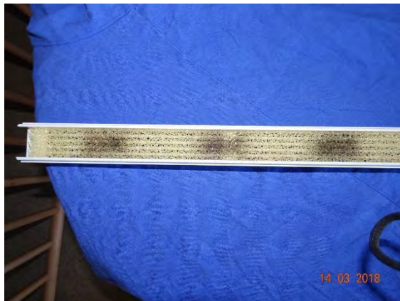
Abbildung 185: WNG ID 810: Zuluftfilter.
