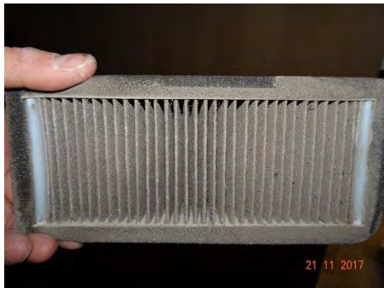
Abbildung 21: WNG ID 110: Zuluftfilter
