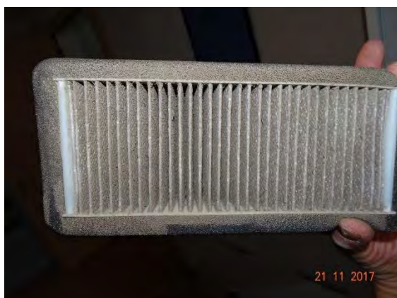
Abbildung 30: WNG ID 120: Zuluftfilter
