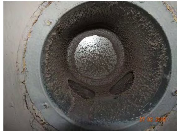
Abbildung 161: WNG ID 720: ABL-Rohr, Bad
